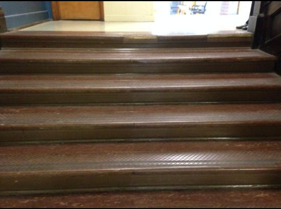
Worn Down Steps
