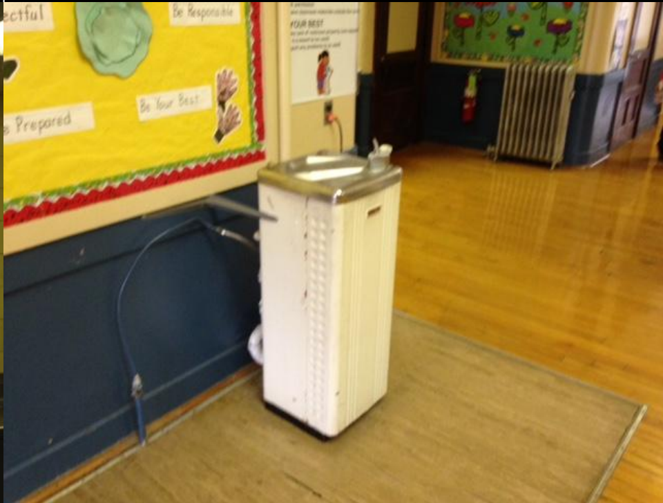
Leaky Water Fountain
